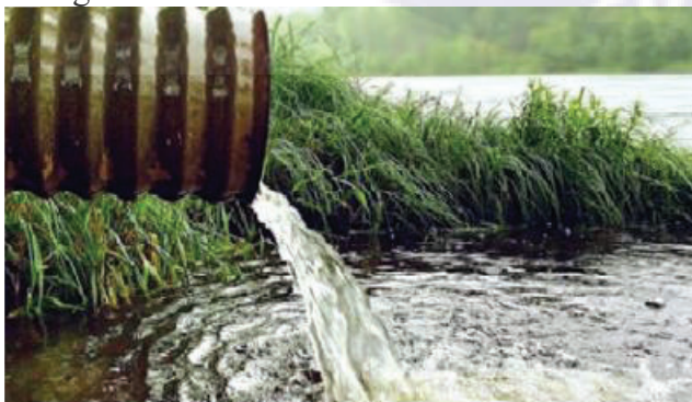
Fig 3: Water discharging into natural body
