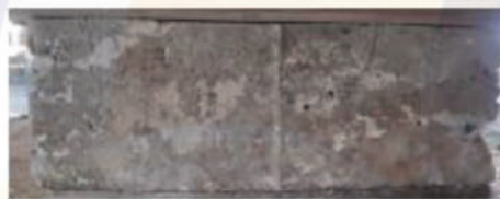
(a) Cracks At Centre
