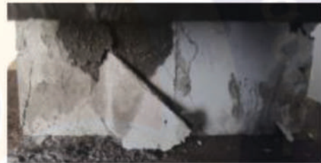
(b) Cracks At Edges
